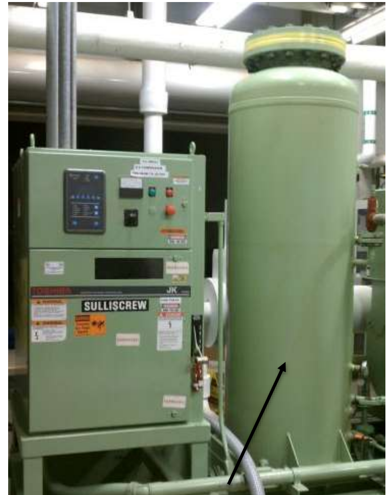
Bulk Oil Separator
