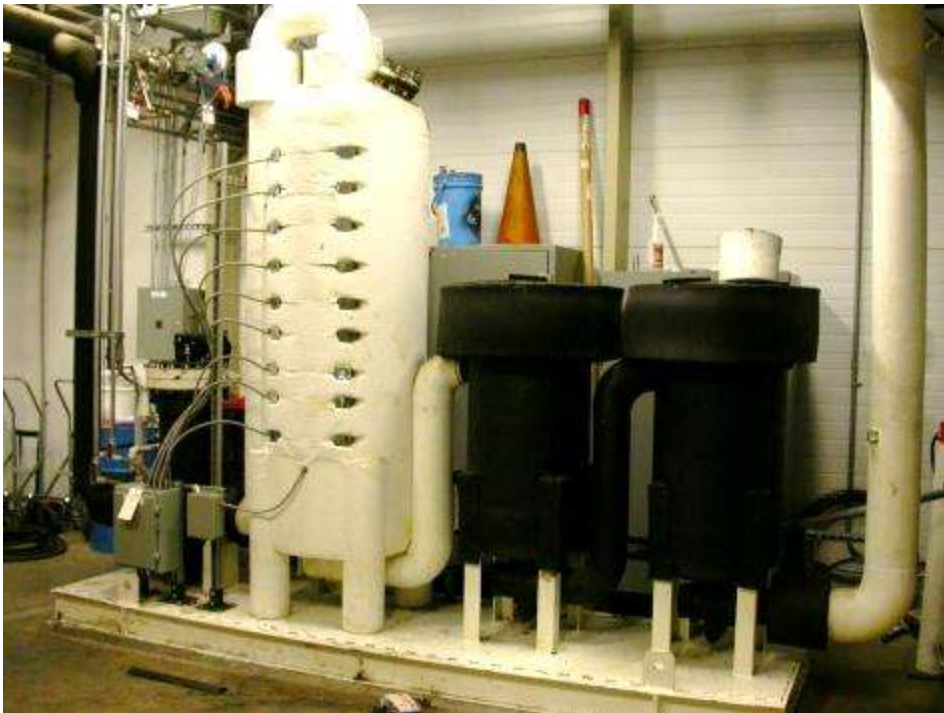
Oil Removal Skid
