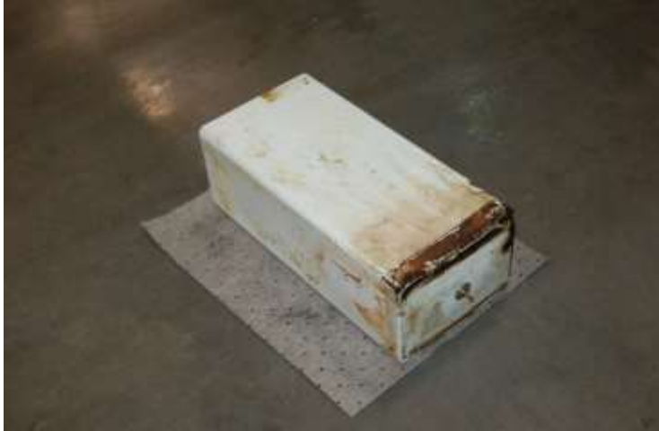
Old 120 kV / 3100 pF GA capacitor (failed)
