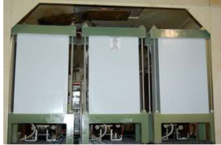
New 150 kV / 3100 pF CSI capacitors with brackets
