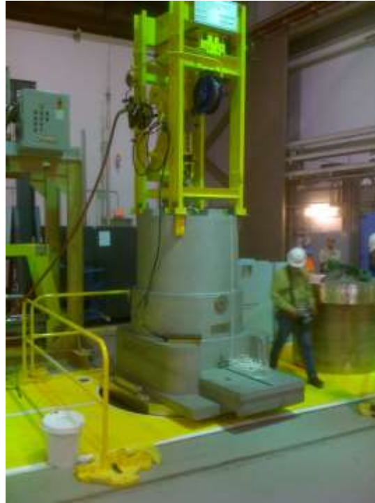
PBW Cask is positioned over Top Loading Port
