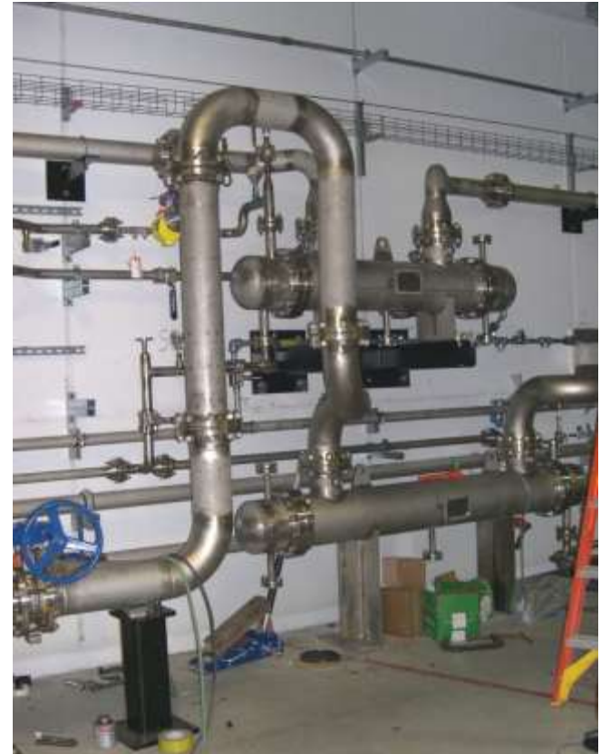
Cooling Loop showing Heat Exchanger Mounted
