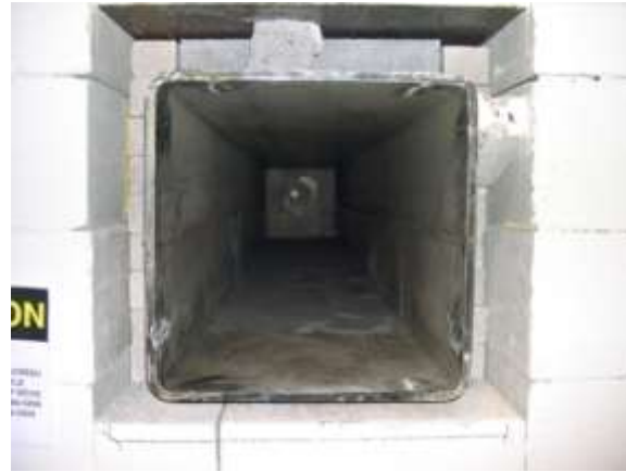
Beam Stop Enclosure
