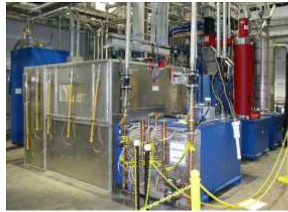
HIGH VOLTAGE CONVERTER/MODULATOR
