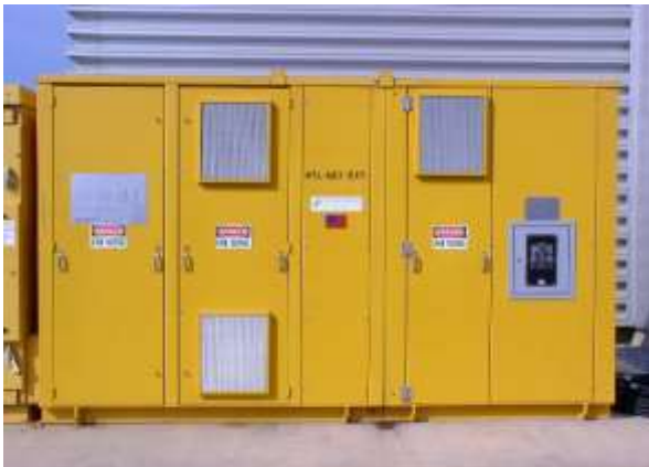
RECTIFIER TRANSFORMER AND FILTERS
