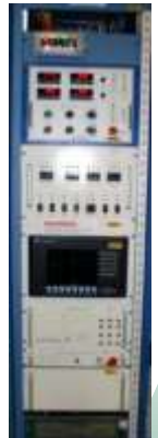
EQUIPMENT CONTROL RACK
