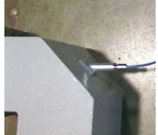
Sensor in waveguide (in Linac tunnel)
