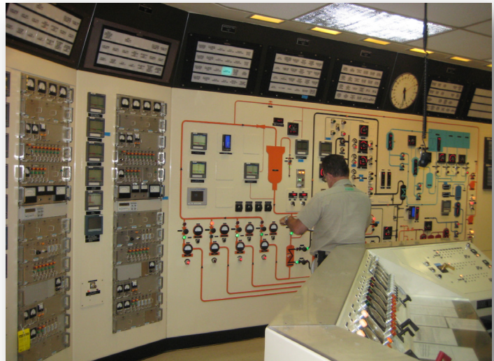
Figure 8: HFIR Control Room
