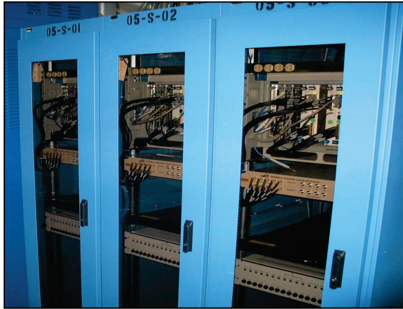
Figure 4.8. The physical layout of the PPU LLRF racks will be similar to that of the existing racks, shown here.
