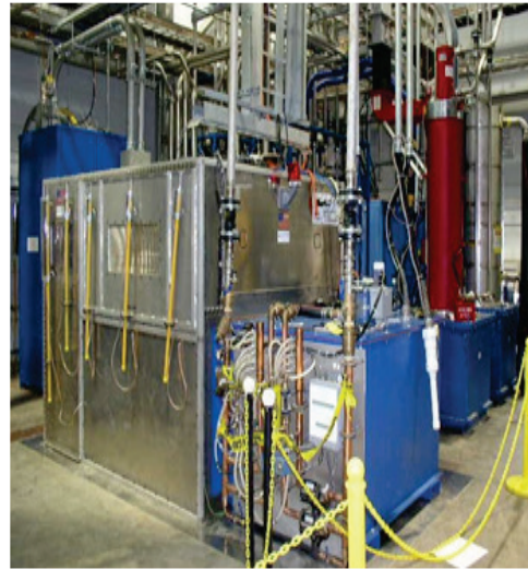
Safety enclosure and oil-filled modulator tank
