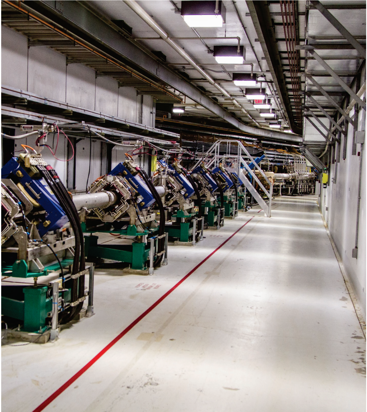
Figure 7.4. Existing RTBT tunnel looking toward the ring. The existing proton beam line is on the left; the stub will connect to the right side of the tunnel.
