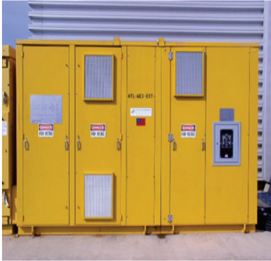
Outside 13.8 kV:2100 V 1.5 MVA transformer
