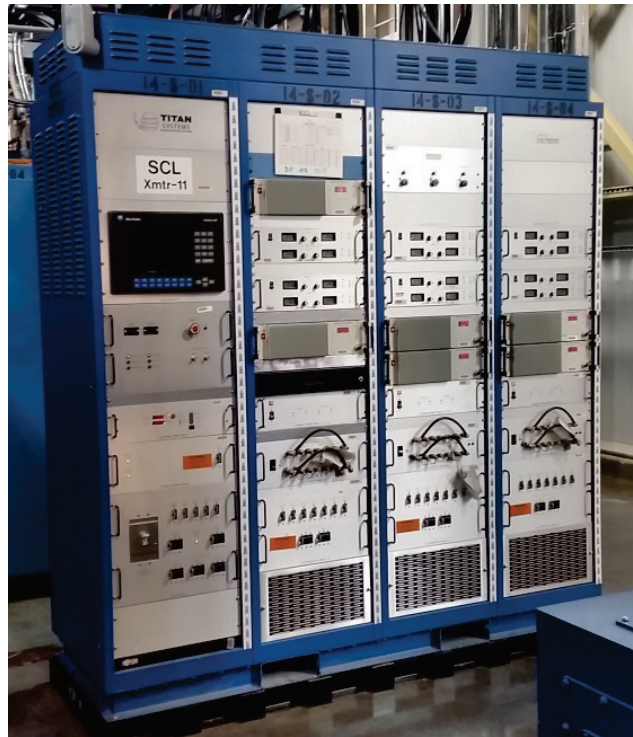
Figure 4.1. The physical layout of PPU RF transmitter racks will be similar to that of the existing racks shown here.
