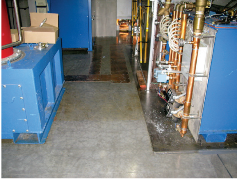
Figure 4.19. Existing ground-plane installation in the klystron gallery.
