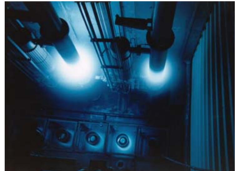
Spent fuel pool →
